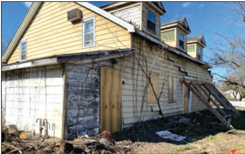
A building on Route 9D building with 'structural deficiencies' was torn down in Wappinger.
