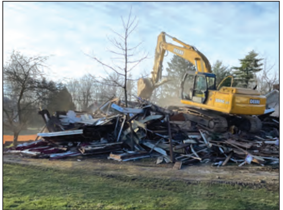
Rubble from a building deemed to have 'structural deficiencies on Route 9D in the Town of Wappinger.
